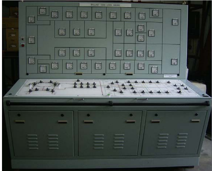
Control panel for ballast tank level gauging
